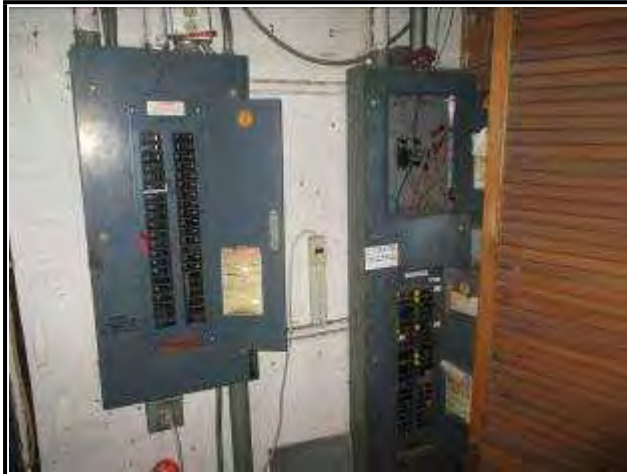
Figure 2.3.3 – Electrical Breaker Panels
