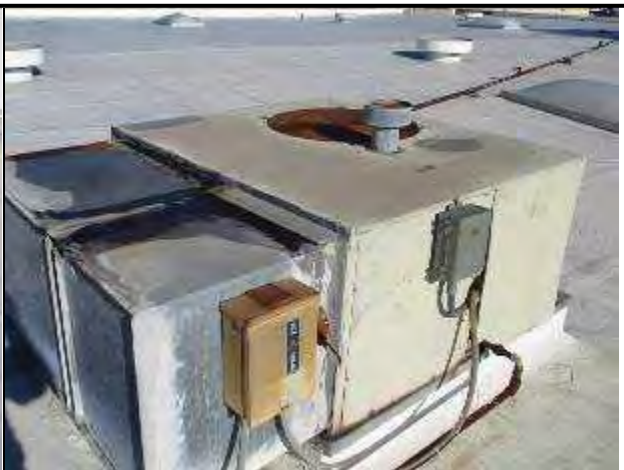
Figure 2.4.2 – Abandoned HVAC unit
