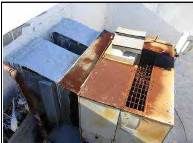
Figure 2.4.1 – Older Day & Night HVAC
