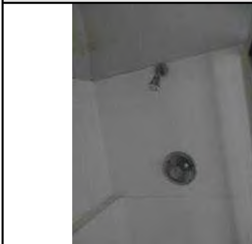
Figure 2.1.5 – Private restroom showerhead
