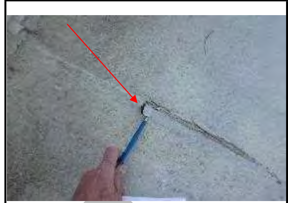
10. Peeling coating at field lap
