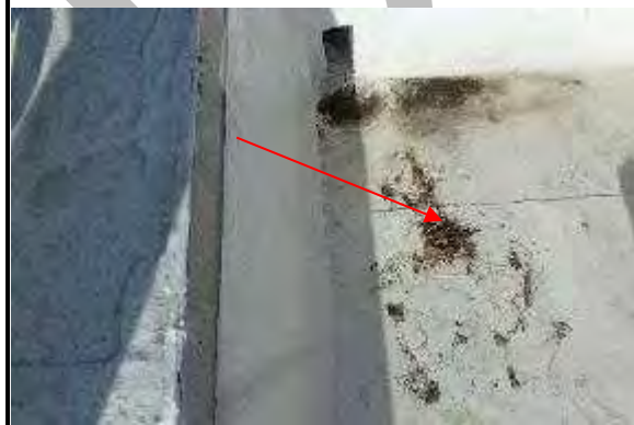
3. Debris on membrane
