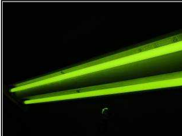
Figure 2.3.5 – Nonfunctional lighting fixtures
