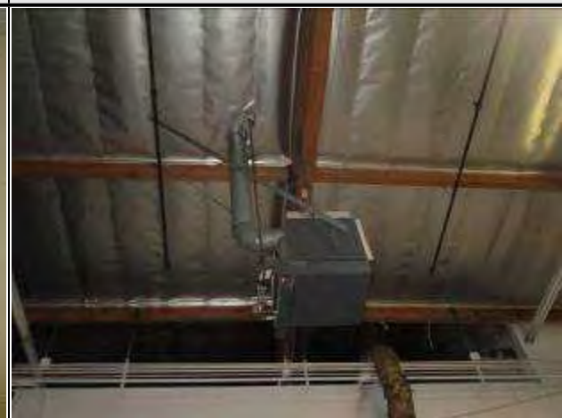
Figure 2.4.4 – Gas Unit Heater
