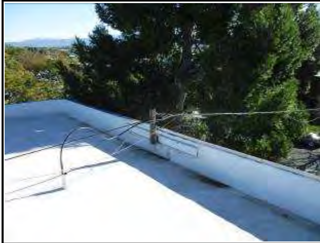
Figure 2.3.1 – Incoming electrical service
