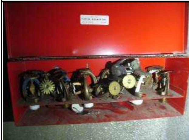
Figure 2.5.3 – Spare sprinkler head box
