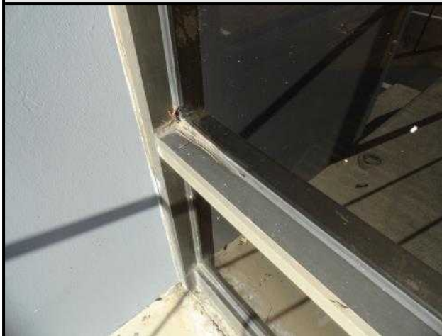
Typical poor condition of glazing gaskets and sealants
