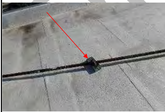
9. Blocking lacks slip sheet
