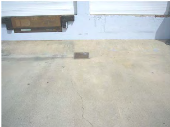
11) View of a typical truck well catch basin.
