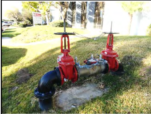
67. Fire sprinkler system detector-check assembly
