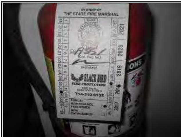
Figure 2.5.1 – Fire extinguisher inspection tag
