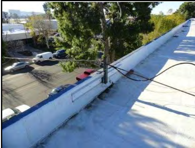
Power for the sub-tenant space at the northeast corner of the building is provided overhead down to electrical panel and main breaker
