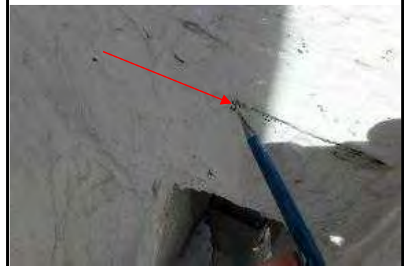
6. Exposed webbing at scupper
