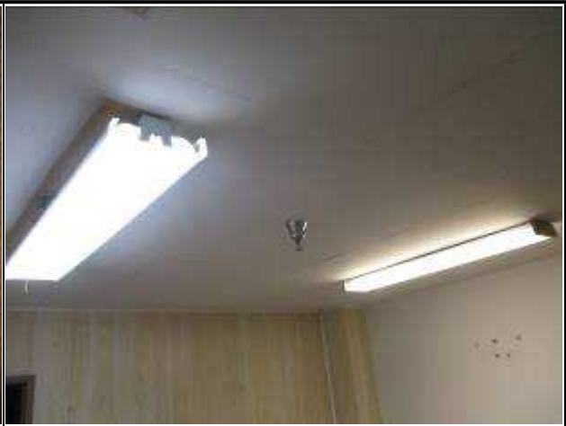
Figure 2.3.4 – Typical T12 fluorescent lighting
