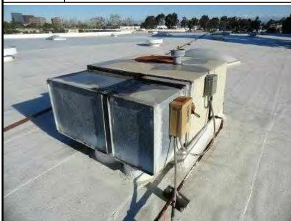
57. Southwest office area gas/electric rooftop unit
