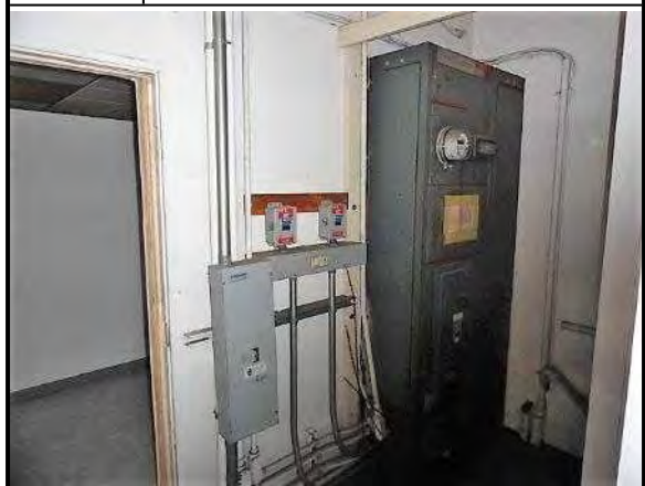
60. General Electric main switchboard, meter and submeters
