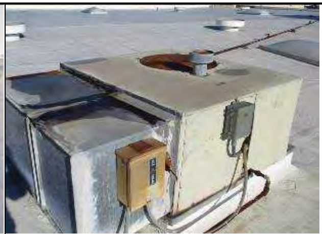
Figure 2.4.2 – Abandoned HVAC unit
