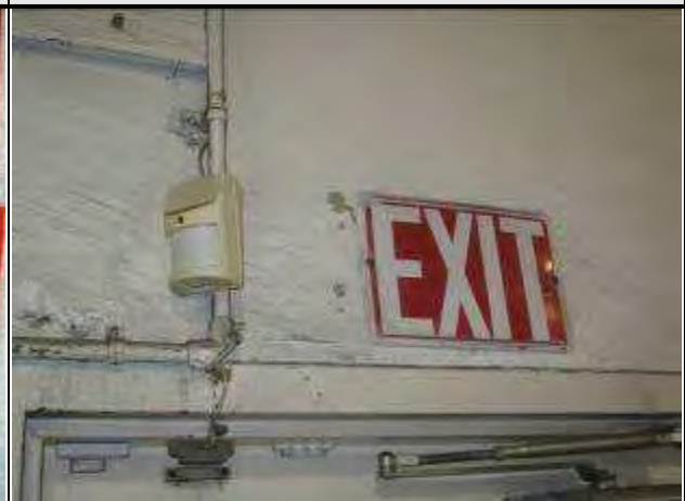
Figure 2.5.4 – Non-illuminated Exit signage
