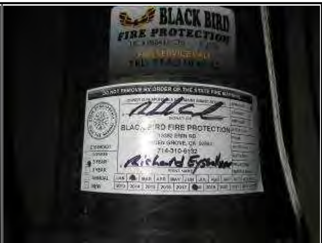
Figure 2.5.2 – Fire sprinkler system inspection tag
