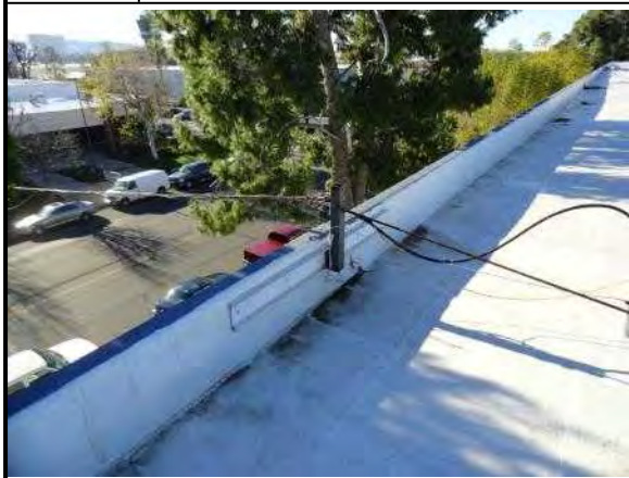
62. Overhead power drop to the switchgear in the northeast office area
