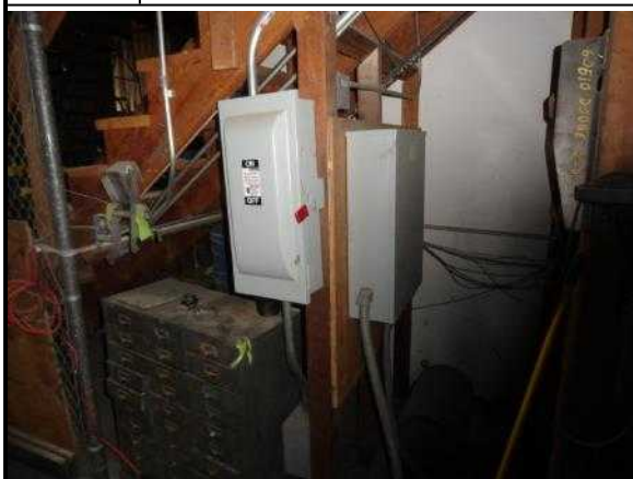
63. Service disconnect serving northeast office area
