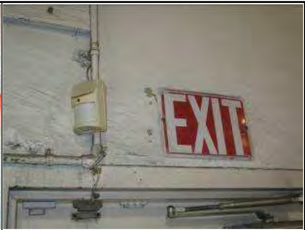
Figure 2.5.4 – Non-illuminated Exit signage
