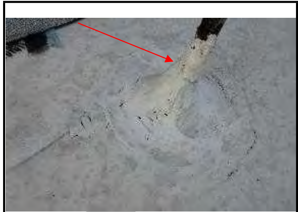
9. Voids in coating at pipe flashing
