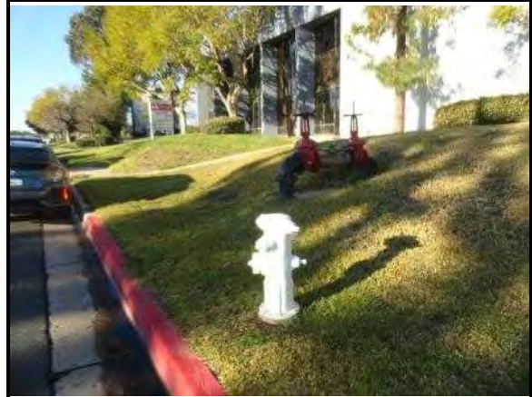
70. Typical fire hydrant
