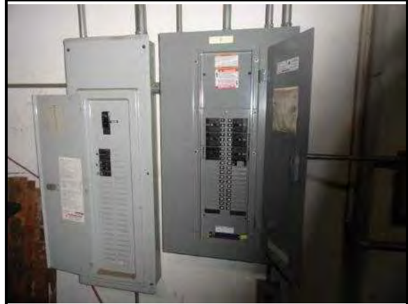
64. Switchgear serving the northeast office area
