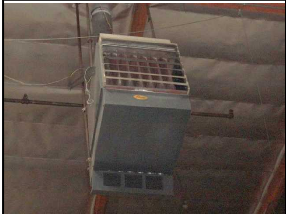
59. Warehouse area suspended unit heater
