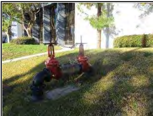
Figure 2.2.1 – Fire sprinkler water piping
