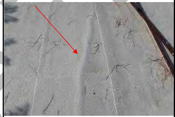
11. Roof membrane ridging
