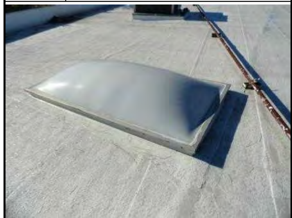
29. Typical skylight has no fall protection
