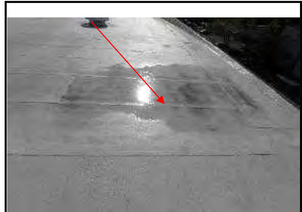
4. Ponding in field
