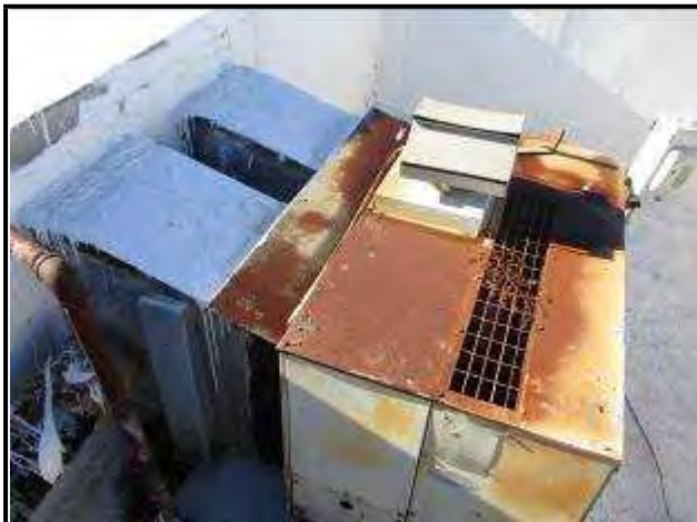
Figure 2.4.1 – Older Day & Night HVAC
