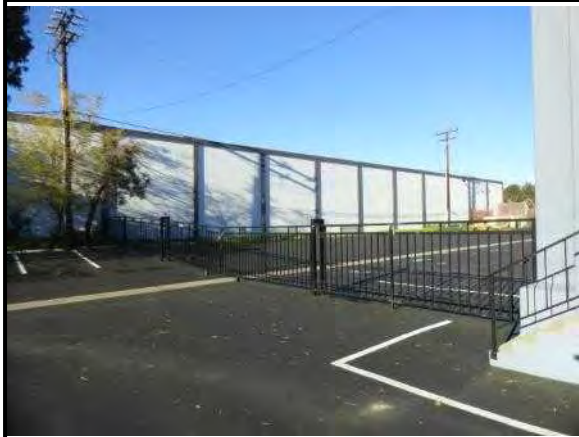
61. Power pole and pole-mounted transformer with feeders underground to the main switchboard in the warehouse
