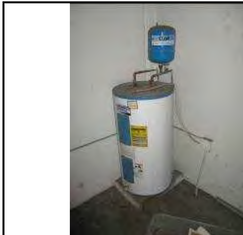
Figure 2.1.1 – Electric water heater
