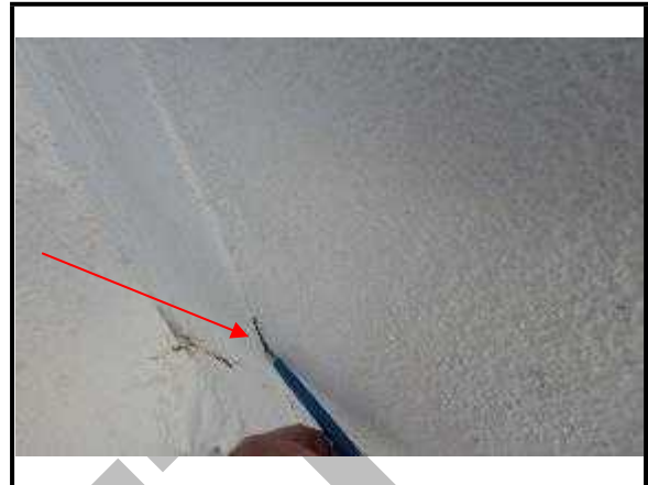
4. Open base flashing seams
