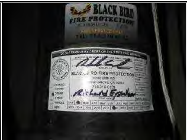
Figure 2.5.2 – Fire sprinkler system inspection tag
