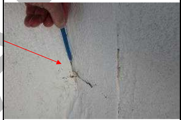
5. Open base flashing seams
