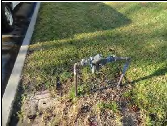
49. Domestic water service meter box and reduced pressure backflow preventer
