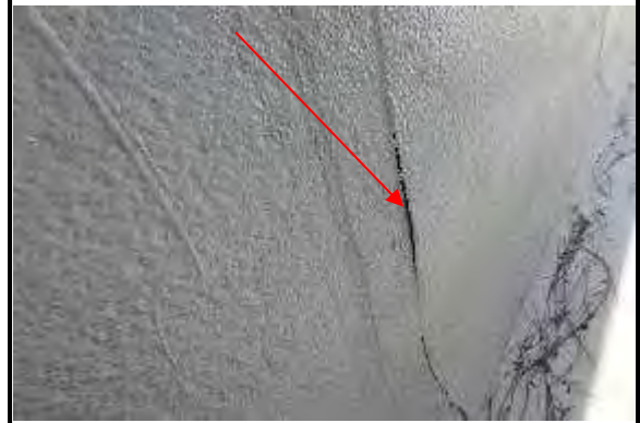
6. Open base flashing seam
