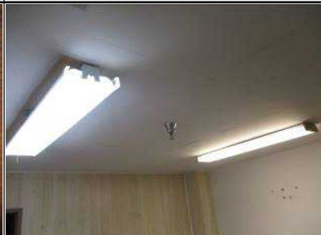
Figure 2.3.4 – Typical T12 fluorescent lighting
