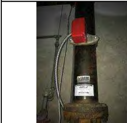
Figure 2.5.5 – Fire sprinkler alarm wiring disconnected
