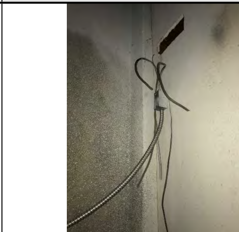
Figure 2.5.6 - Fire sprinkler alarm wiring disconnected
