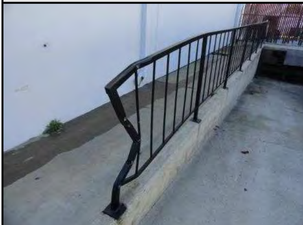
Damaged railing at northeast corner exterior loading dock
