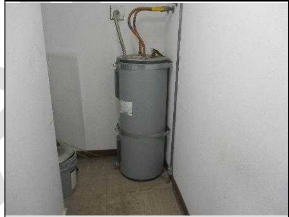
11. Hot water heater in south east office portion with seismic straps.
