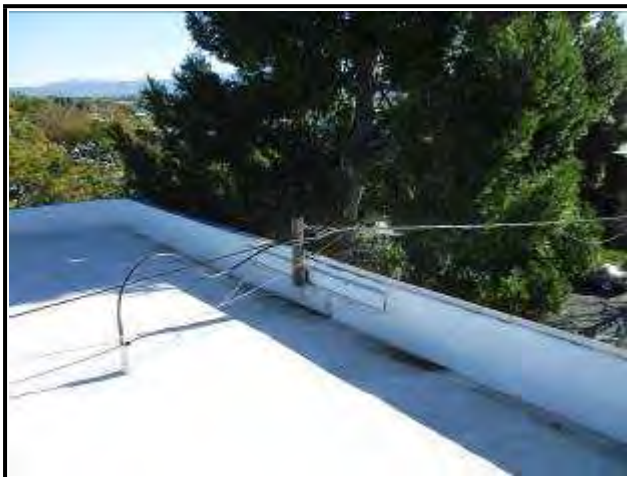
Figure 2.3.1 – Incoming electrical service
