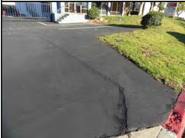
Asphalt paving condition showing seal coating applied over incomplete crack repairs
