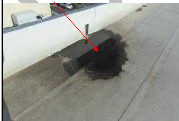
3. Ponding in field
