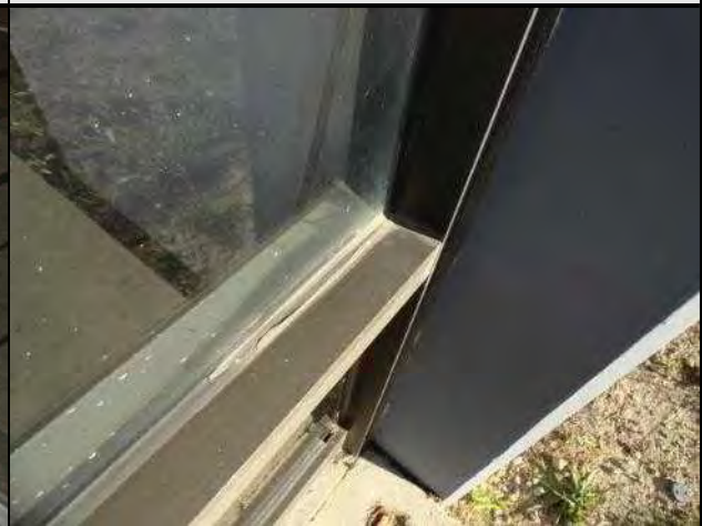
Typical poor condition of glazing gaskets and sealants
