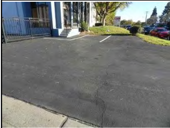
13. Typical asphalt paving condition showing improperly repaired cracks before seal coating
