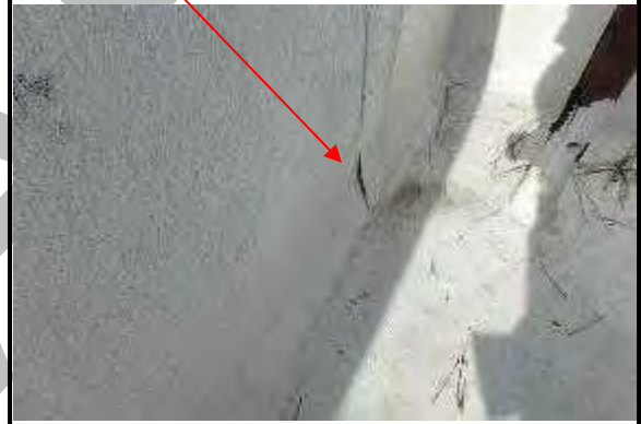
5. Open base flashing seam
