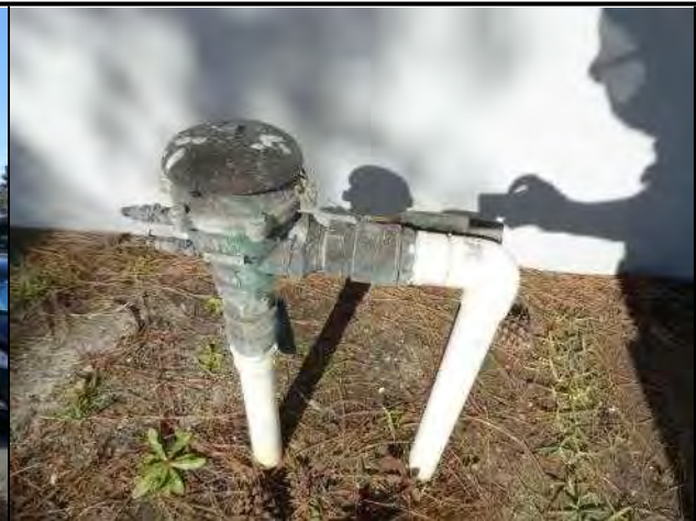
Landscape irrigation system backflow preventer view
