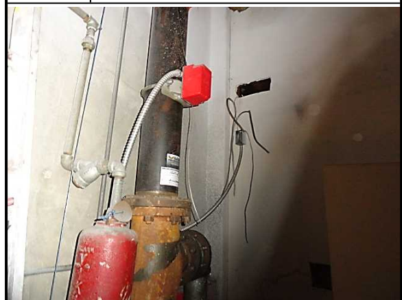
66. Fire riser showing disconnected flow switch
