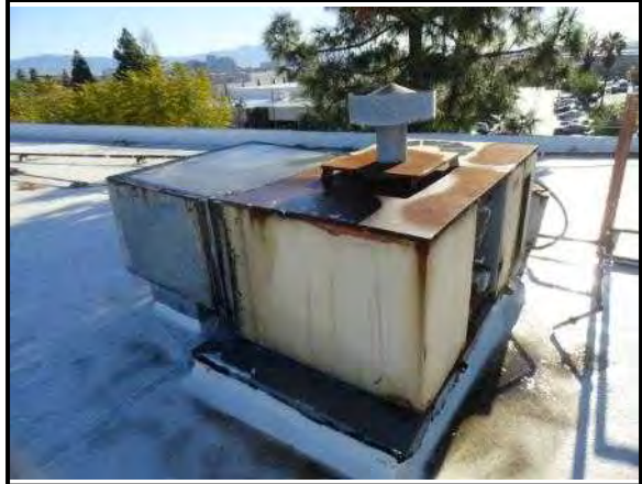
58. Southwest office area gas/electric rooftop unit
