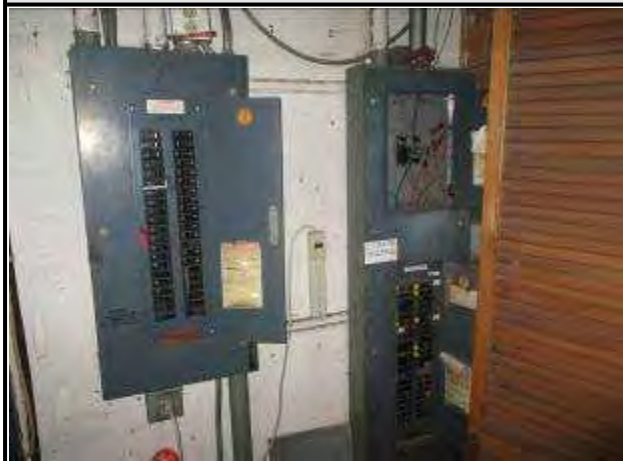
Figure 2.3.3 – Electrical Breaker Panels
