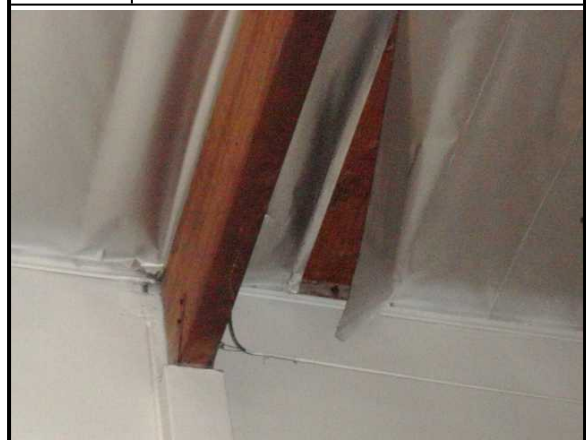
36. Typical structural framing at the exterior wall and pilaster with no seismic hold down bracket upgrading evident
