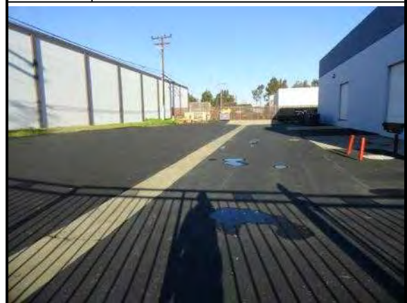
11. Parking spaces were previously striped along the west side of the building but not restriped after sealcoating
