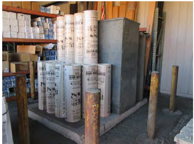
28. View of a pad-mounted transformer located on the subject property.
