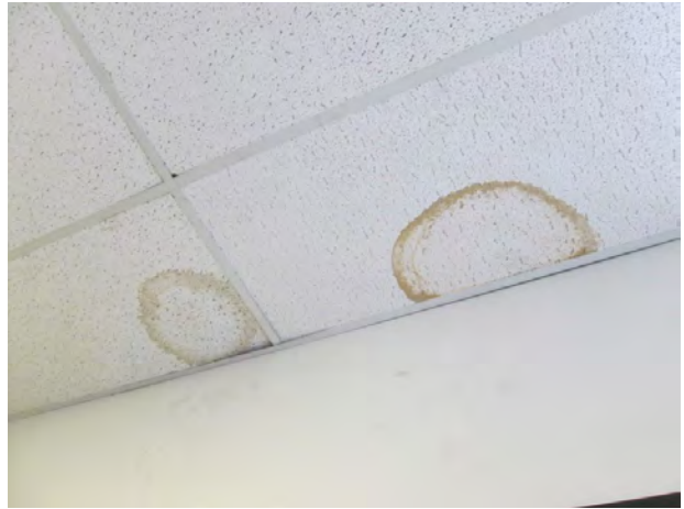
26. View of minor water-staining on the ceiling tiles in the operations office located on the northwestern portion of the subject property.
