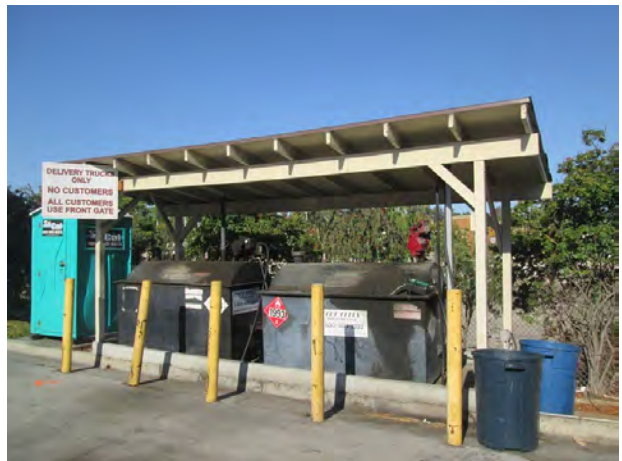
24. View of two approximately 300-gallon diesel ASTs located on the northwestern portion of the subject property.
