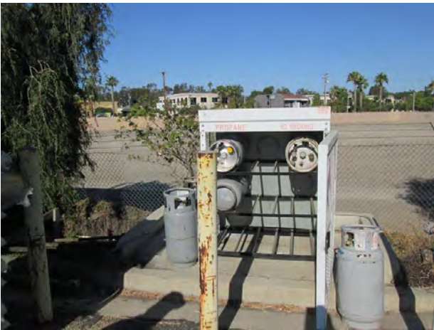
27. View of the propane tank storage area located on the northern portion of the subject property.
