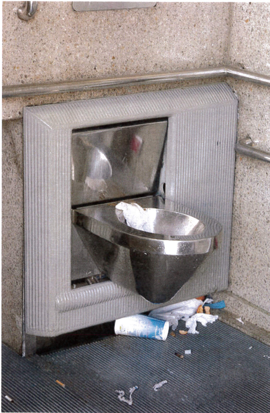
The inside of the restroom near City Hall before cleaning contains all manner of detritus: hypodermic needles, condoms, excrement and assorted trash. Photo by Jason Winshell/SF Public Press.
